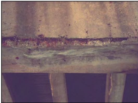
Figure 138. Spall in Pier 2 cap beam. Location 1.
