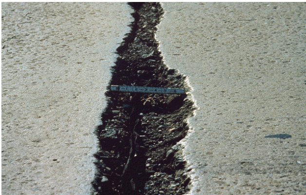
Figure 132. Deck spalling along joint. Location 2.
