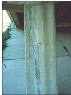
Figure 139. Crack in Pier 3 column. Location 3.
